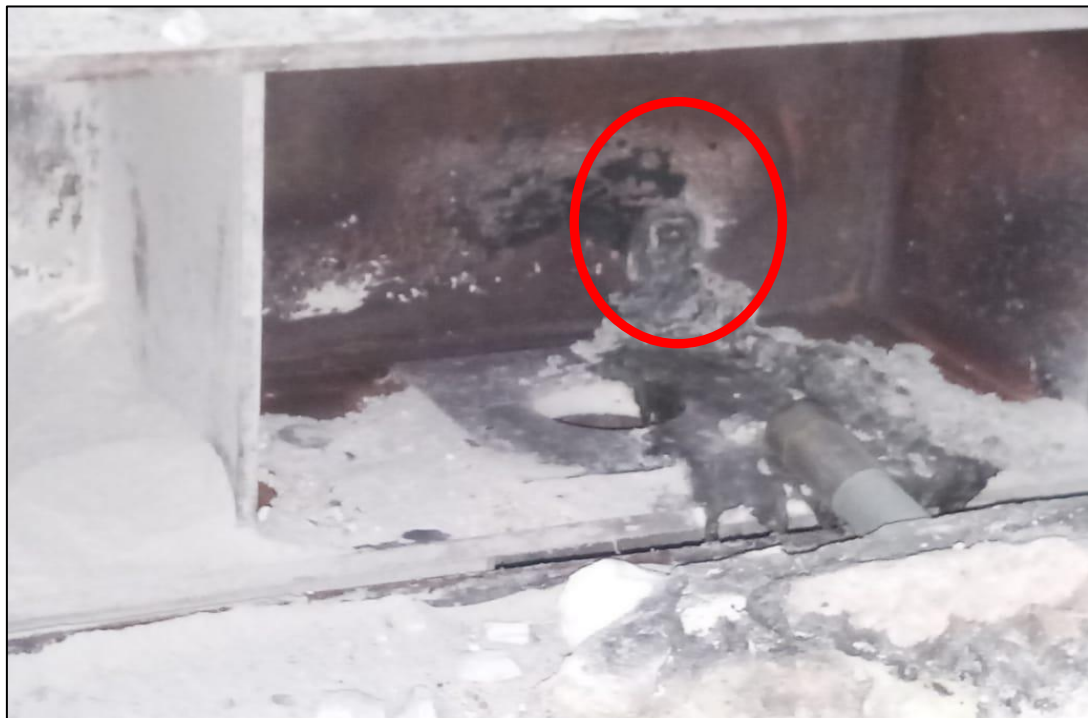
Figure 7. Pot leakage from side shell through hot spot.
